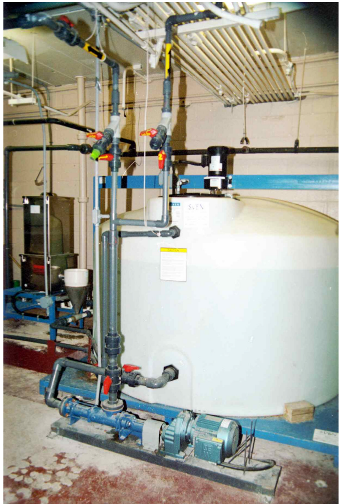
Pictured in the background left is a SVENMIX.D 3325. In the foreground right is an 1100 gal. tank with a SVENMIX LS Mixer. The system automatically makes a 0.15% polymer solution on demand. An ultrasonic level controller in the tank initiates the process. The solution is fed to a belt thickener by the PC pump next to the tank.
